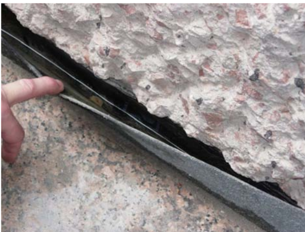
Insufficient height at the waterproofing finish against a vertical element as well as lack of adherence thereunto. Immediate corrective measures must be adopted.
