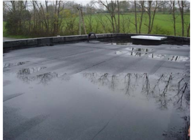
Roof on which waterlogging occurs.
