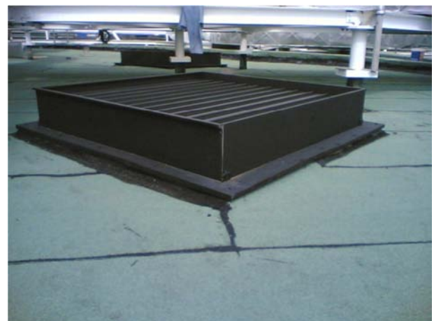
Waterproofing joint against a vent which is not very high. Immediate corrective measures must be adopted.
