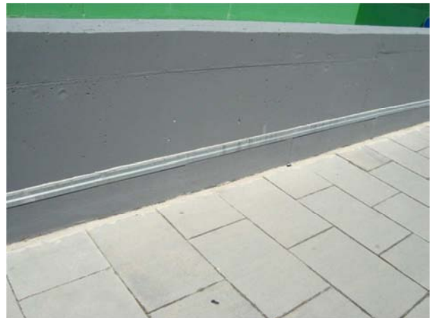
Waterproofing finish against an upstand with the correct height. The finishing profile is properly installed and sealed above.
