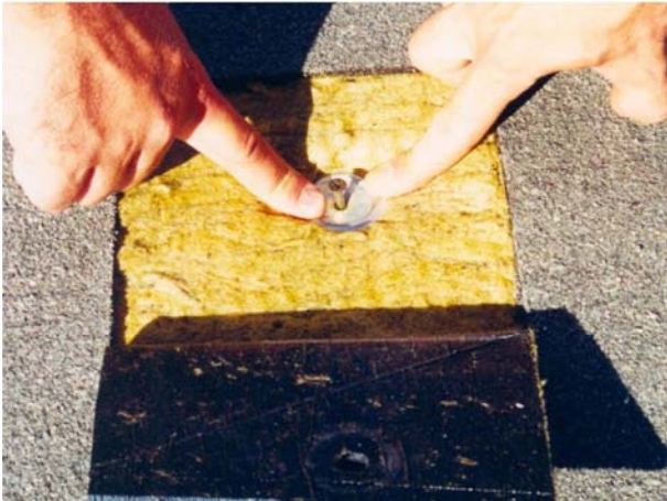
Inappropriate affixation that has brought about the puncturing of the waterproofing system.
