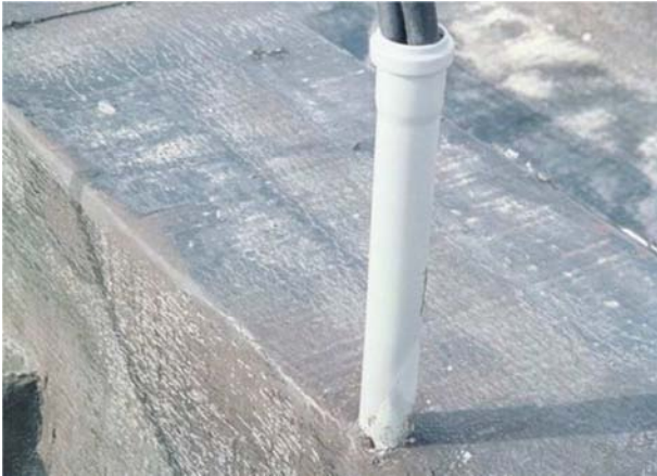
Waterproofing finish with duct channels without suitable special parts.
