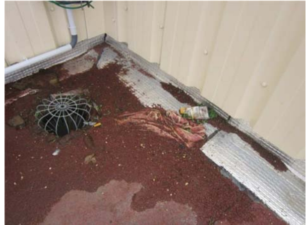
During site inspections check for any debris which may be found on the roof and see to its removal.
