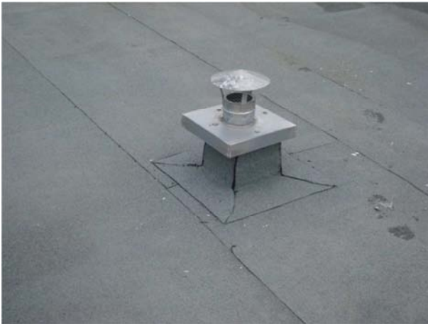
Passage of vent ducts through conduits.
