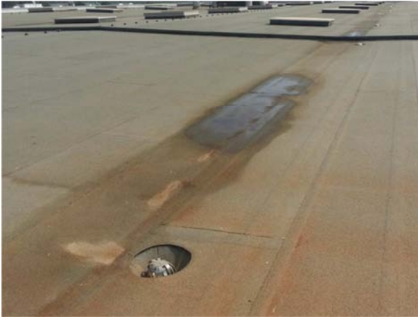
Channel with water accumulations in the vicinity of the gutters.
