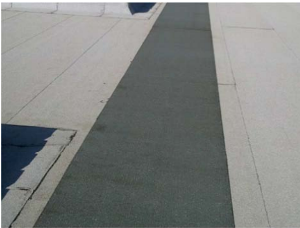
Detail of a maintenance corridor welding to the autoprotected waterproofing ESTERDAN PLUS 50/GP TECHNICAL CORRIDORS.
