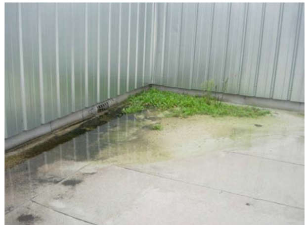
Condition of the roof in a building near areas with a lot of vegetation on which no periodic site inspections have been carried out.
