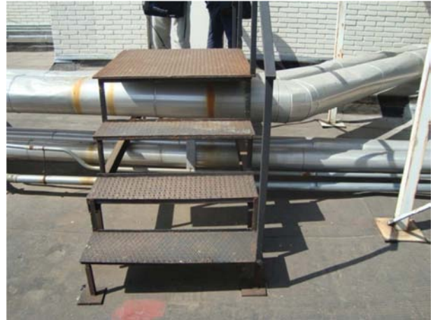
Supporting of elements on the waterproofing without any protection element. Immediate corrective actions must be adopted.
