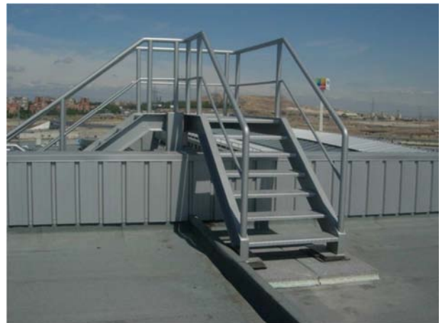
Metallic stairs support by means of reinforcement elements to avoid damage to the waterproofing membrane.
