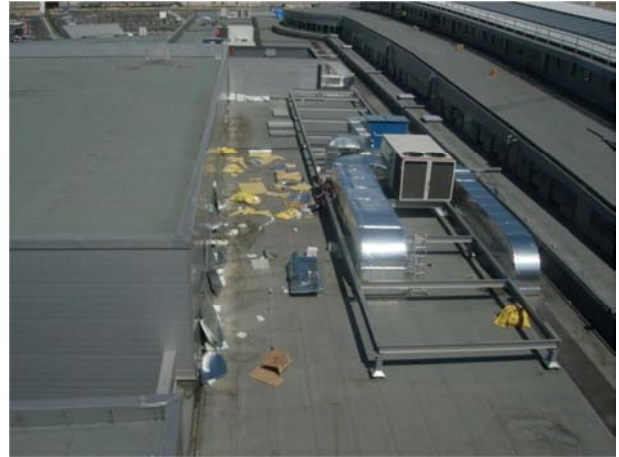
The installation of equipment on the roof may bring about serious damage to our waterproofing system.
