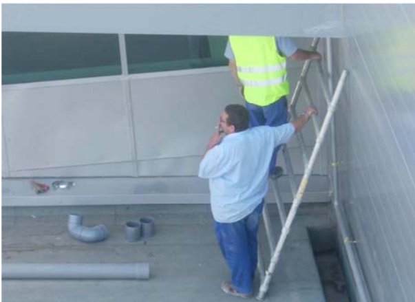
Works in areas adjoining the roof may bring about damage thereunto, particularly in the case of autoprotected roofs.
